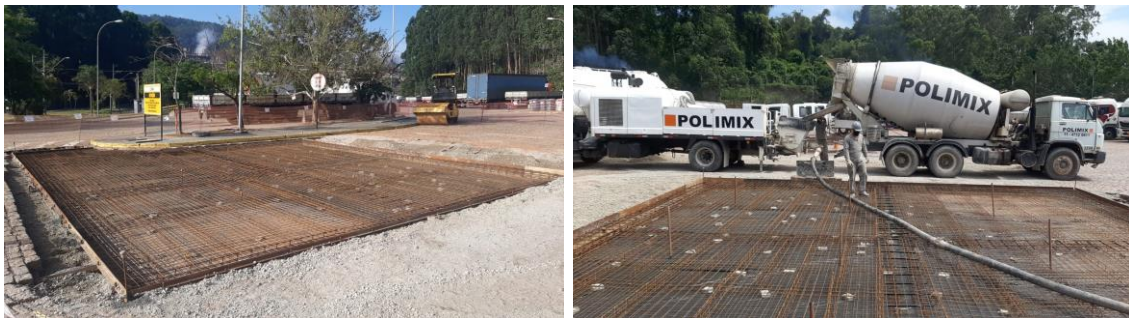
Figure 2. Preparation of the jointed plain reinforced pavement: side formwork and steel reinforcement (left); concrete mixing truck, concrete pump, and pipeline used to conduct the concrete from the pump to the placing site (right).
