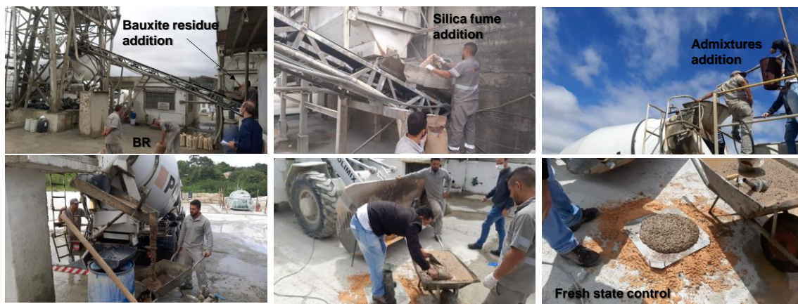
Figure 3. Illustration of the stages of addition of bauxite residue, silica fume, and superplasticizer into the concrete. Below, it is shown the moment when a portion of concrete is collected from the truck for fresh state evaluation.
